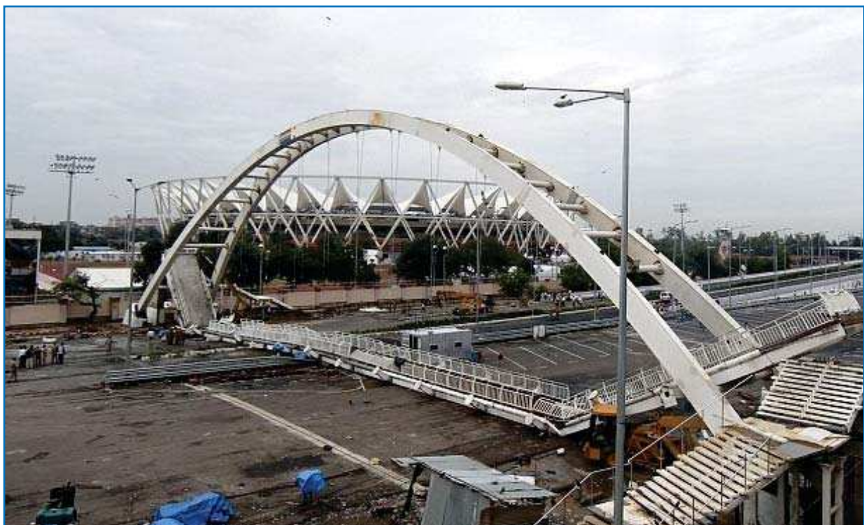
Collapsed FOB near JLN Stadium
