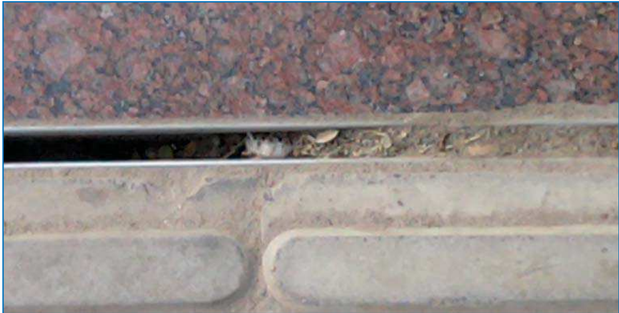
Choked polymer drain
